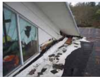
Water floods Palmdale Presbyterian Church in Jeanne's wake
